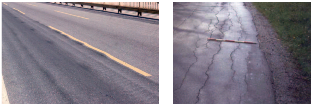
Figure 1. Damage of flexible pavements by rutting (left) and fatigue failure (right)
